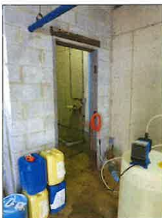
Corrosion on door frame
