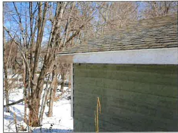
Paint on eave trim in poor condition and no gutter present
