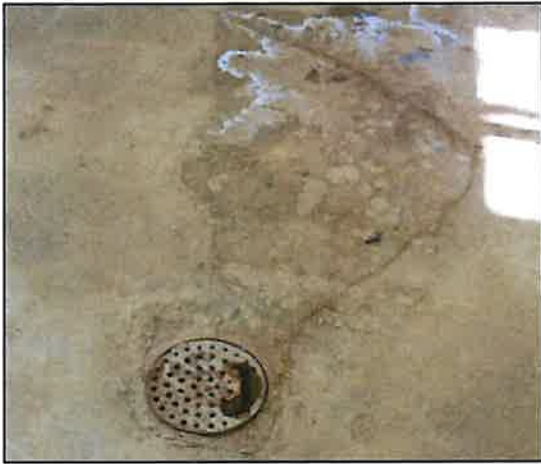
Evidence of Past Chemical Spills to Floor Drain
