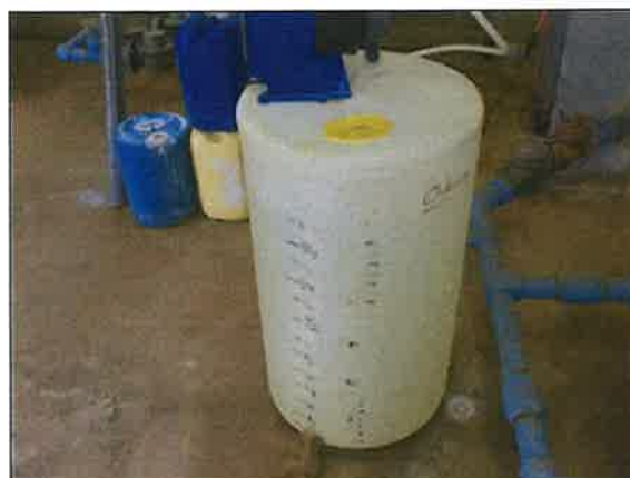
Chemical tanks lack labels
