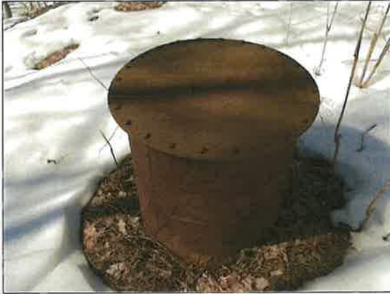
Access Manhole Cover Bolted to the Frames
