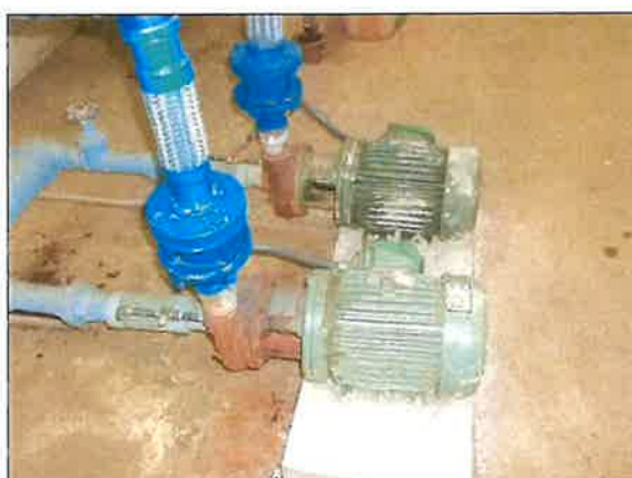
Heavy Corrosion on Water End of Booster pumps
