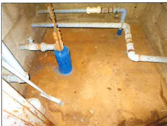
Deterioration of concrete floor slab in old chlorine room
