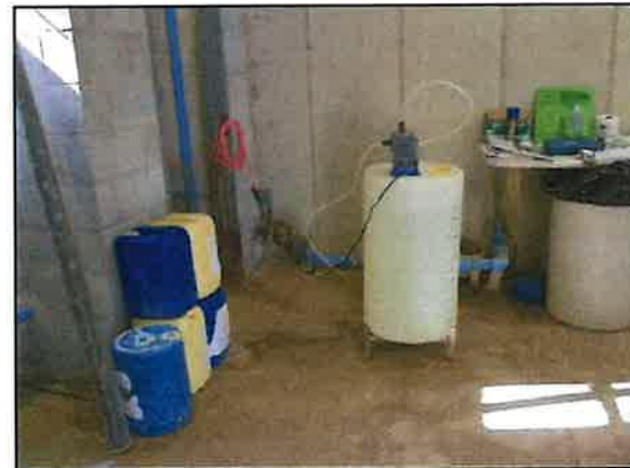
Metering pumps plugged into extension cords; new receptacle should be provided
