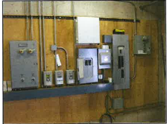
Electrical Equipment inside Wellhouse/Treatment Building
