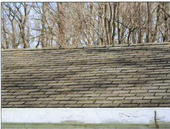
Deteriorated Asphalt Shingle Roof
