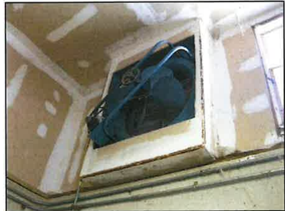
Exhaust fan – original to facility
