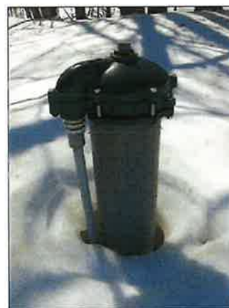
Well 3 lacking level instrumentation and labeling
