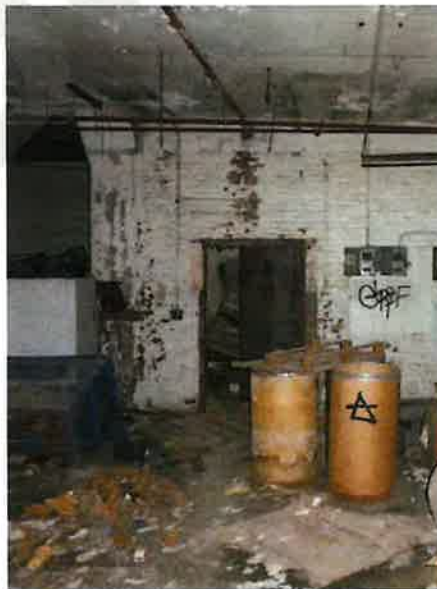
^ Debris and deterioration on the south building
